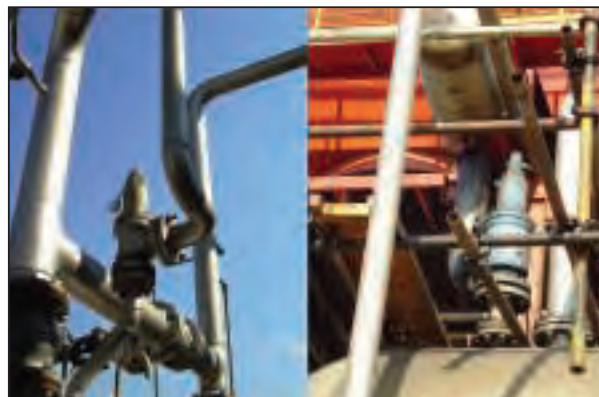
FIGURE 3. Non-free-draining lines in installed relief lines, such as shown in these two constructions, may cause accumulation of liquids that can hamper relief valve performance
